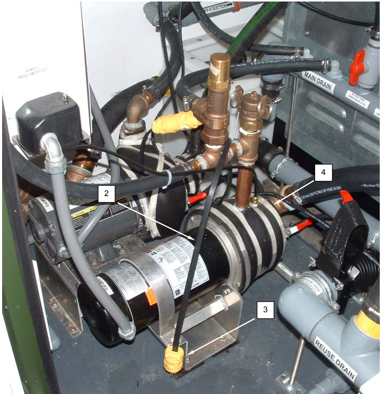
Figure 3. Replace the Heat Tapes.
