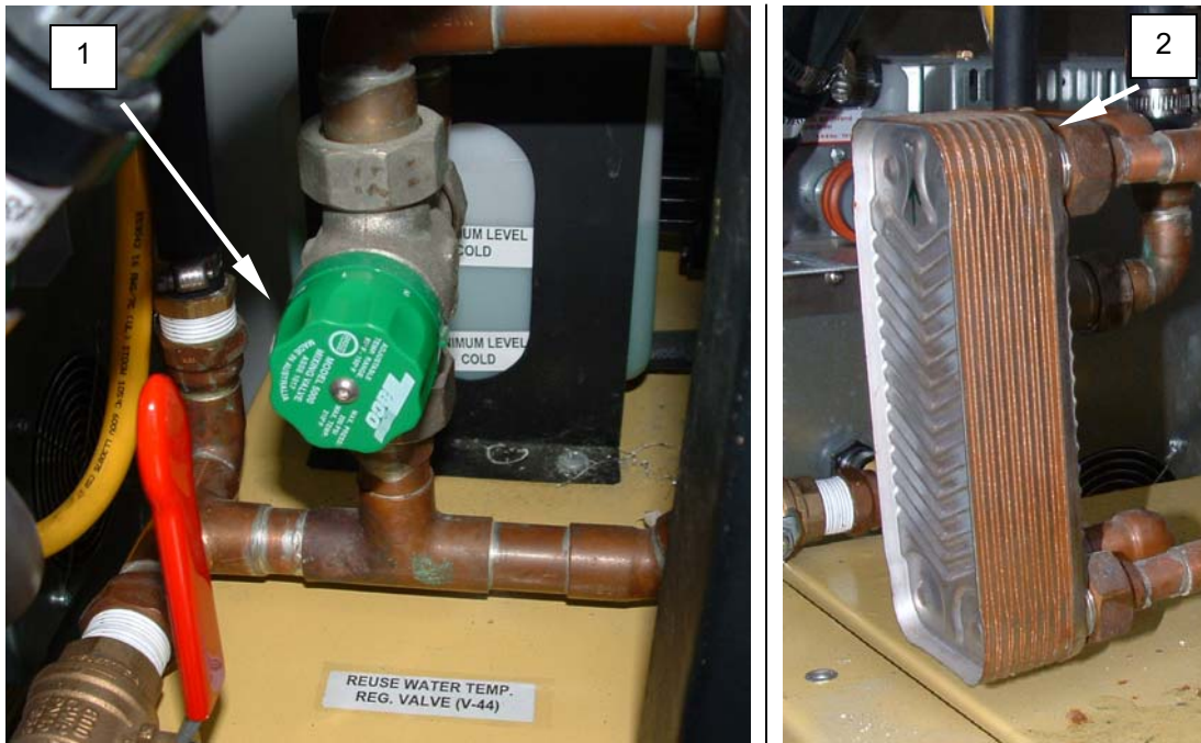
Figure 5. Boiler Operating, doesn't Heat Reuse Water.
