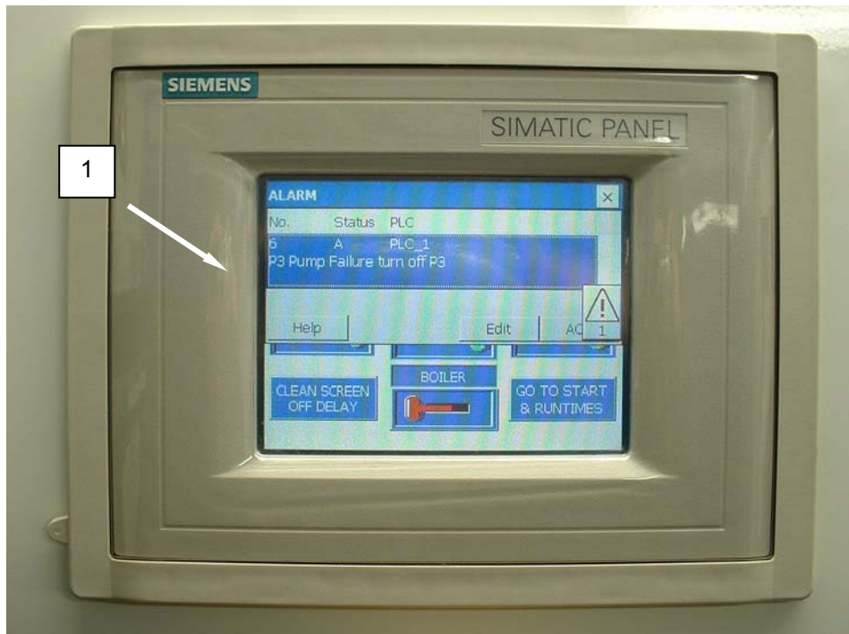
Figure 20. P3 Pump Failure Alarm on PLC Display.
