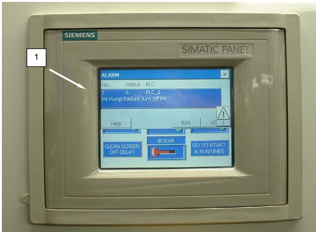
Figure 22. P4 Pump Alarm on PLC Display.
