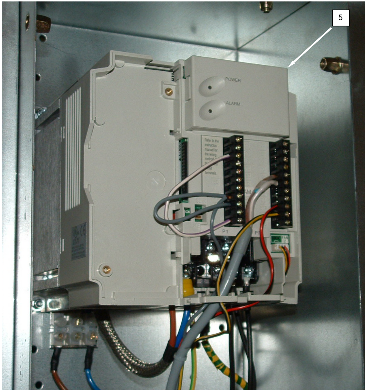
Figure 4. Replace the Washer Variable Frequency Drive.
