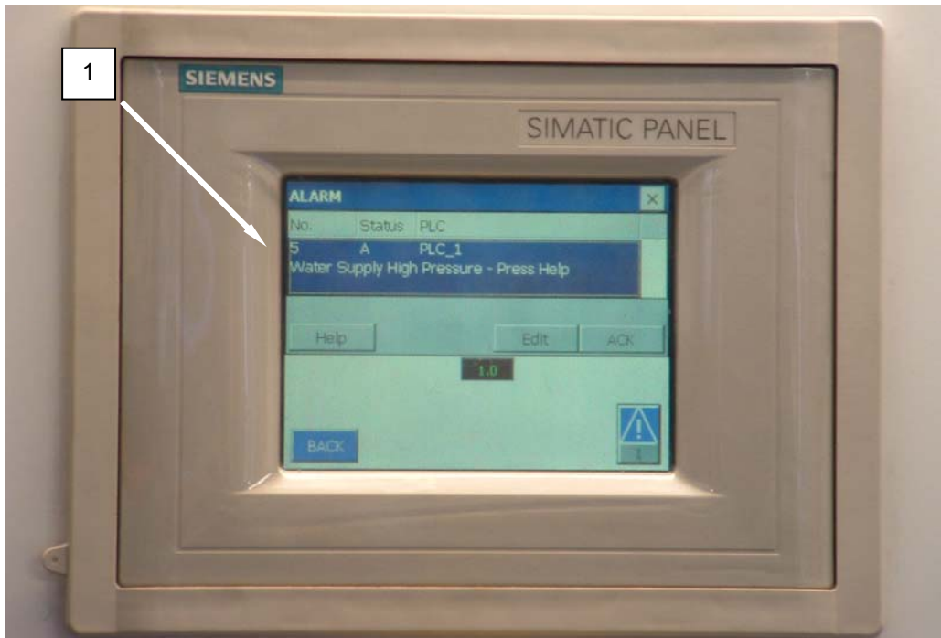
Figure 3. Water Supply High Pressure on PLC Display.
