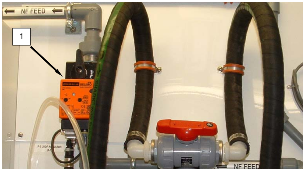
Figure 4. Actuator Valve A-1.
