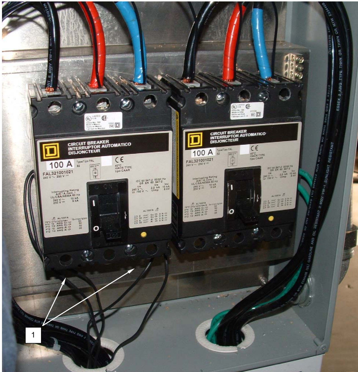
Figure 4. Test Circuit Breakers – Dryer Panel.
