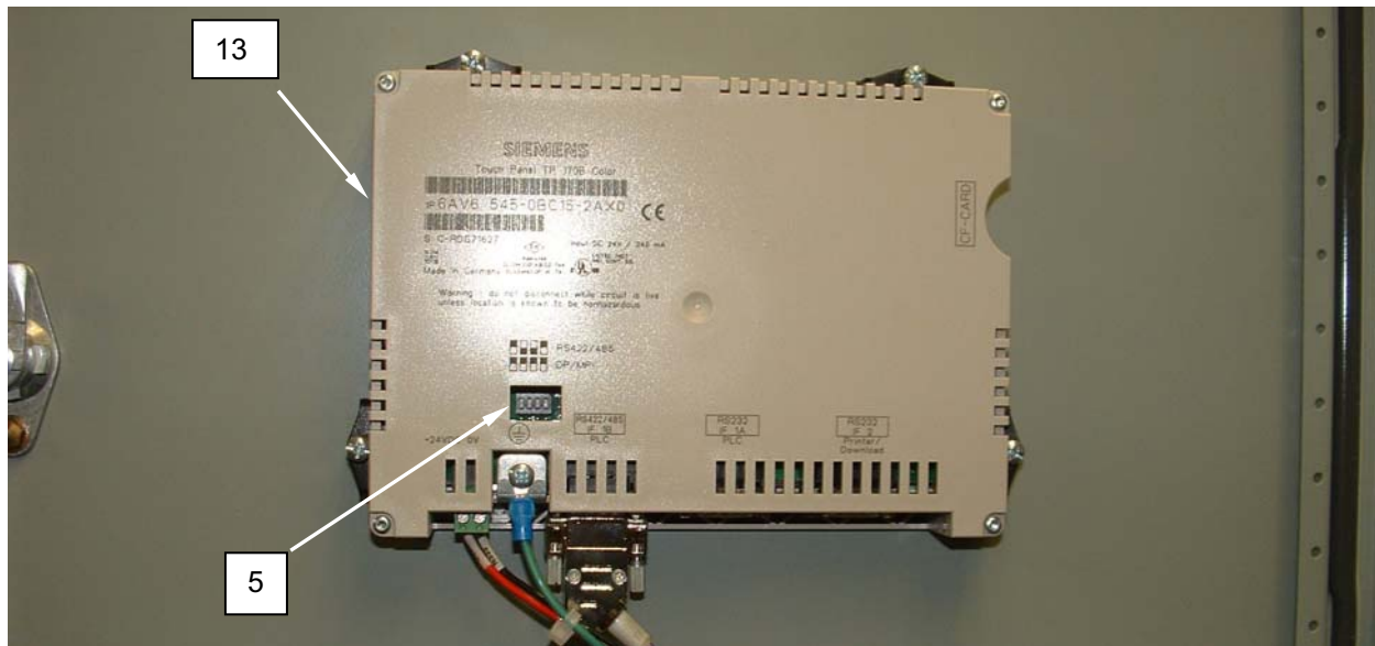
Figure 7. Replace Human Machine Interface (HMI).
