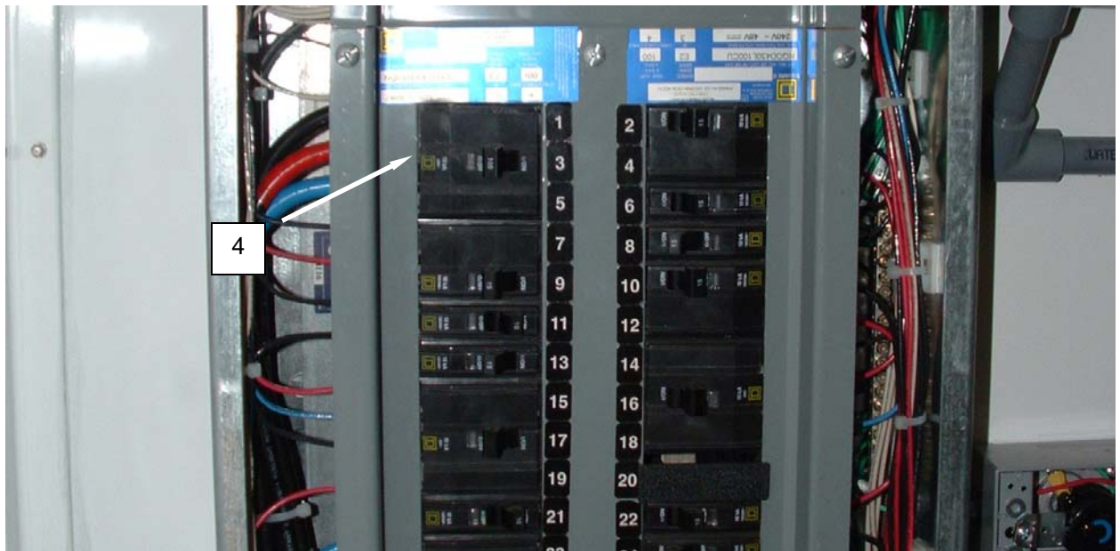
Figure 2. No Electrical Power to any Equipment.
