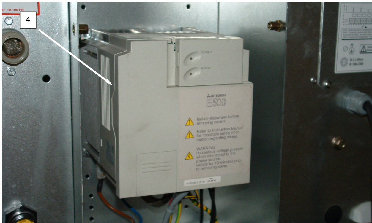
Figure 3. Replace the Washer Variable Frequency Drive.
