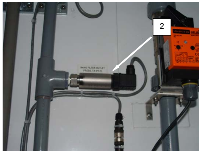
Figure 16. Nano Outlet Pressure Sensor Failure Alarm on PLC Display.
