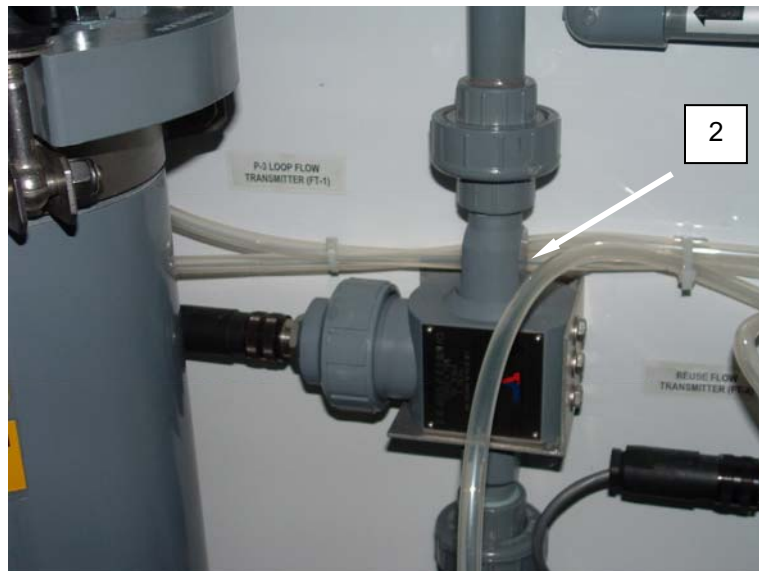
Figure 13. P3 Loop Flow Sensor Failure Alarm on PLC Display.
