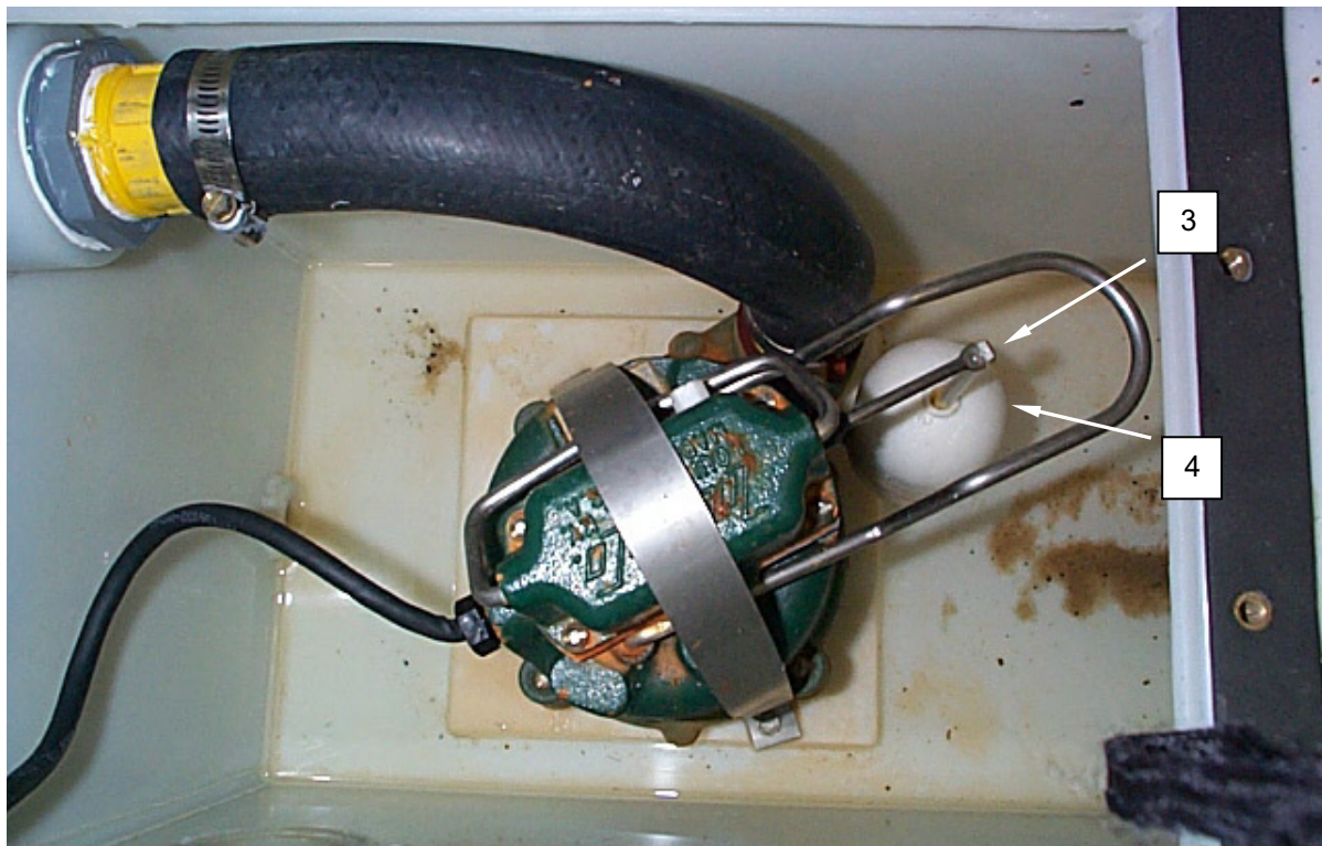
Figure 1. Test the Drainage Tank Pump Float.
