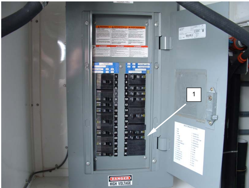
Figure 1. No Electrical Power to Equipment.
