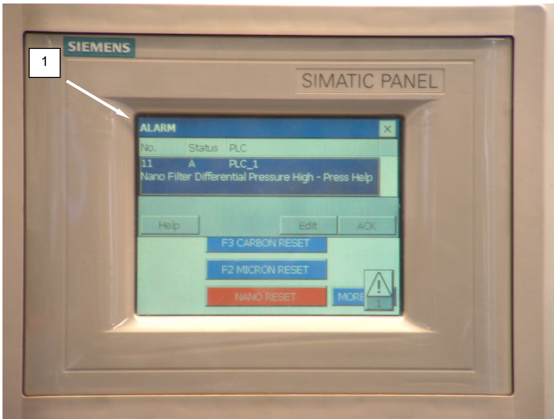
Figure 18. Nano Filter Differential Pressure High Alarm on PLC Display.
