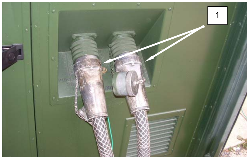
Figure 1. No Electrical Power to Equipment.
