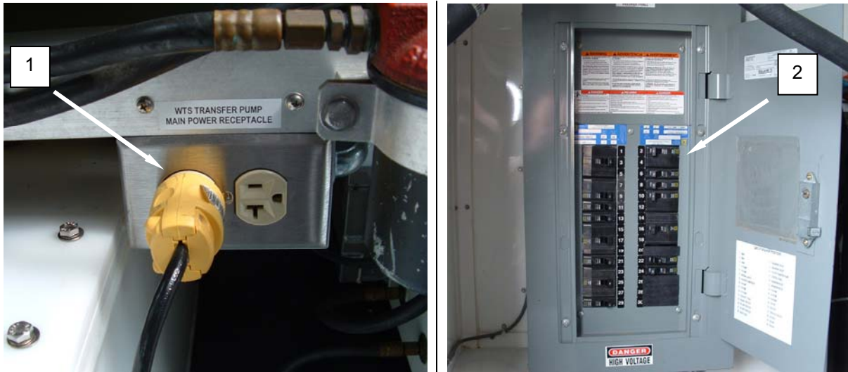
Figure 5. Check Pump and Circuit Breaker.
