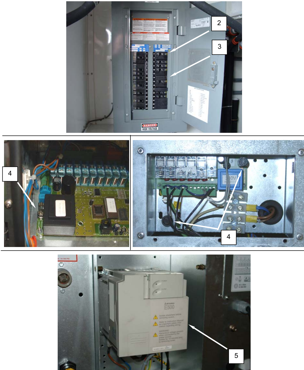
Figure 2. No Electrical Power to Washers.
