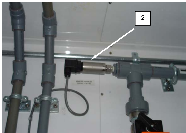
Figure 17. Nano Inlet Pressure Sensor Failure Alarm on PLC Display.
