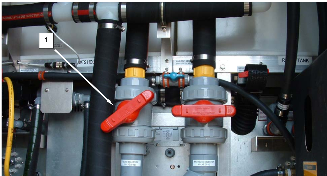
Figure 2. WTS Hold Tank Overflows.
