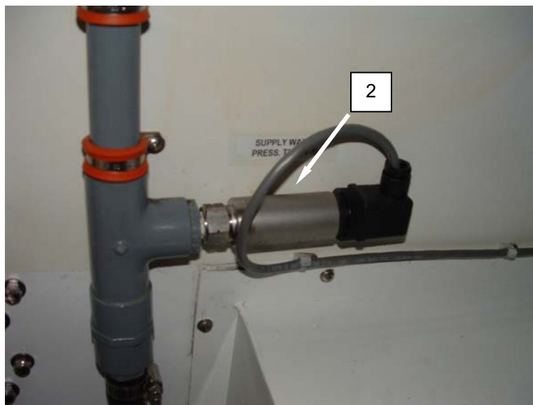
Figure 2. System Pressure Sensor Failure on PLC Display.
